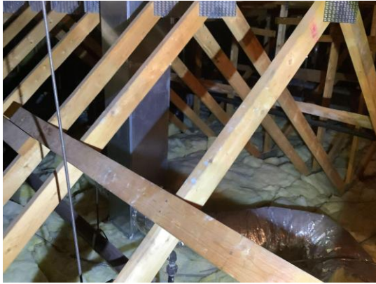
H7 - Ducts are above the insulation. While some have insulation (likely R-6), the supply coming down from the RTU on the roof does not.
