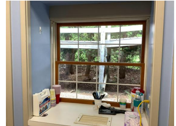
BE11 - The single pane windows in the Community Room are candidates for replacement.
