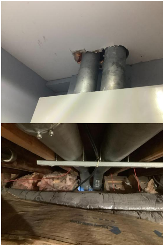
BE7 and BE8 - Conduit runs through the ceiling of Room 112 and you can see from the attic there is a significant gap that allows air leakage. Spray foam and/or stuffing fiberglass insulation around this conduit would block this air loss.
