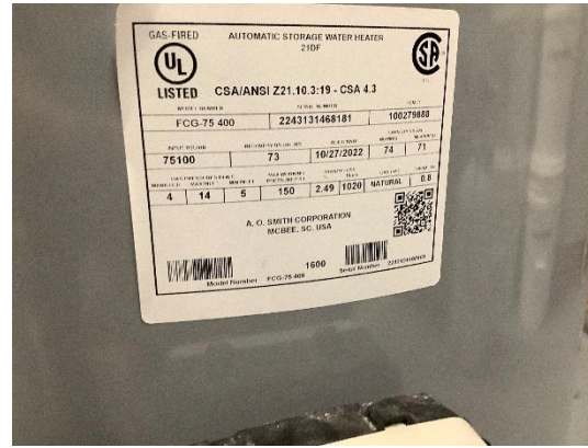
H9 - The label for the main hot water heater (75 gallon, gas) states it was manufactured in October 2022.
