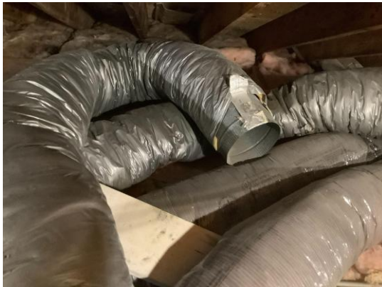
H8 - This duct has been disconnected. When your HVAC contractor comes for their next service visit, have them connect this.
