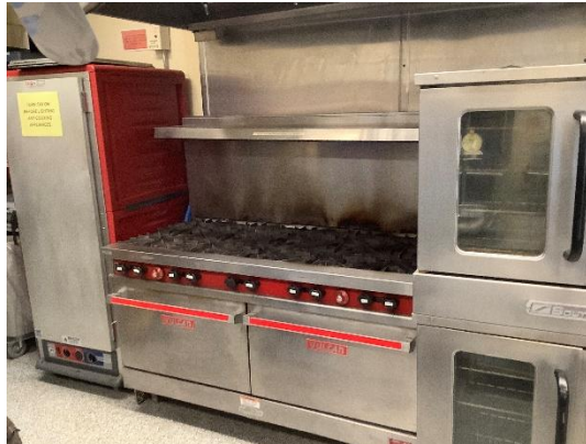
E16 – The pilot lights on this gas range use a surprising amount of gas!
