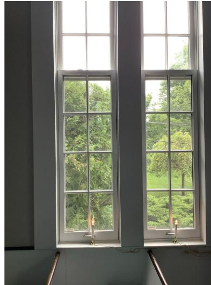
BE9 - The chapel has high quality Pella thermopane windows.
