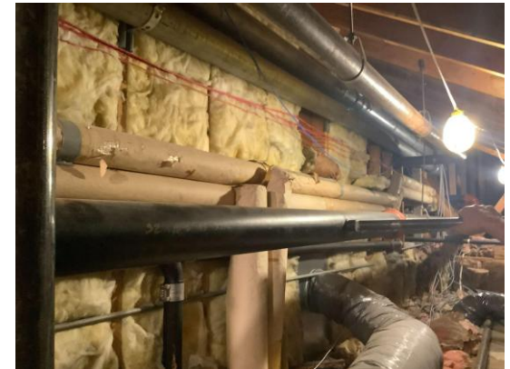
BE5 — Note the insulation removed from one of the stud bays toward the middle of this photo.
