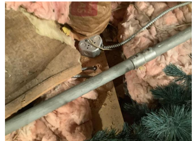
BE6 — The insulation does not fit against the joist, leaving a gap. Note also an electric line running through a hole drilled in the joist that hasn't been filled with spray foam.
