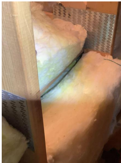
BE4 — The Narthex ceiling is a difficult shape to create a continuous insulation layer and shows gaps in the original installation.
