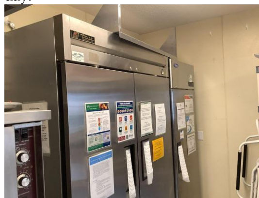
E4 — True refrigerator and Atosa freezer in the kitchen
